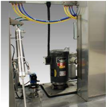
▶ Pump for Agitation and Filtration
